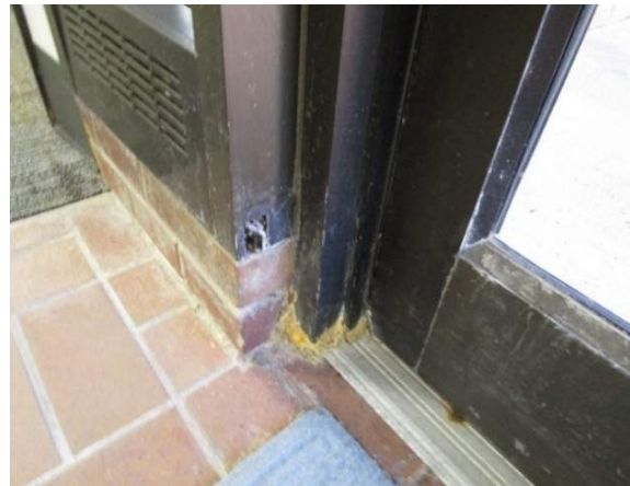
Corroded Aluminum Door Frame
