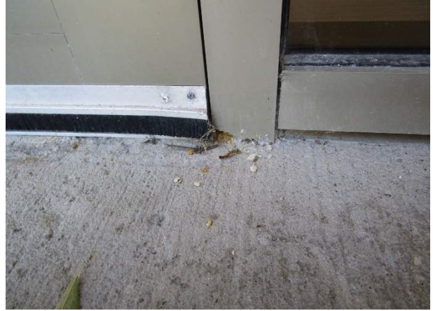
Corrosion of Door Frame
