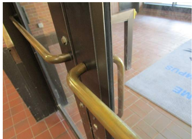
Worn Push Bars Interior Doors E108
