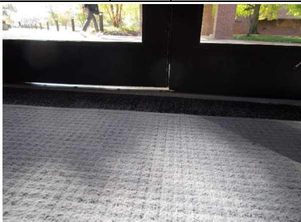
Air Gap Under Door
