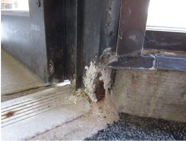
Corroded Frame at Door T102
