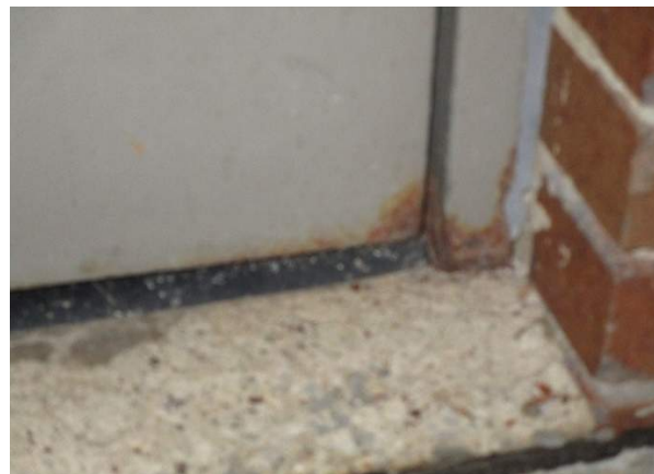
Rusted Door and Frame
