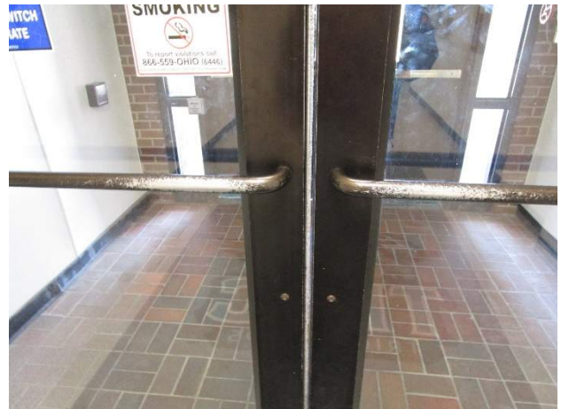
Worn Hardware Exterior Vestibule C100D East
