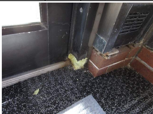
Corroded Door Frame
