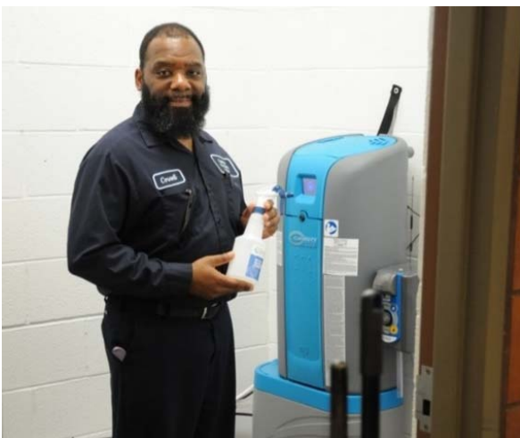
Building Services worker Cornell Murray with the ionized water treatment system at the Eastern Campus
